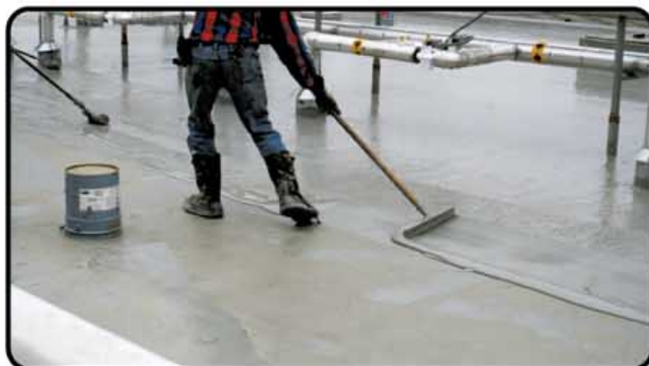
The renewal process will save you money and extend the life of your roof
